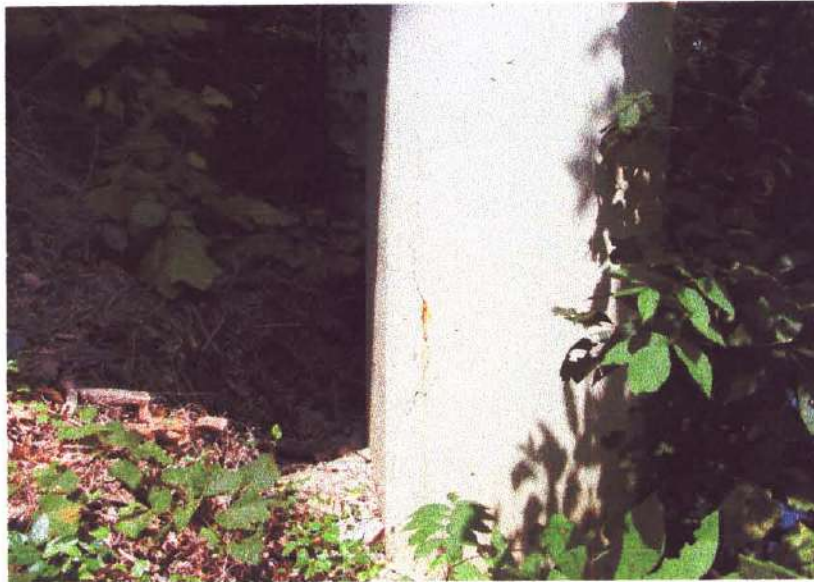
CRACKS IN COLUMN "C", BENT NO. 1
