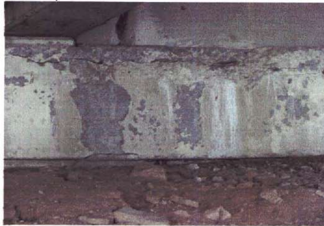
Spall @ Lt. Side of Abutment No. 1
