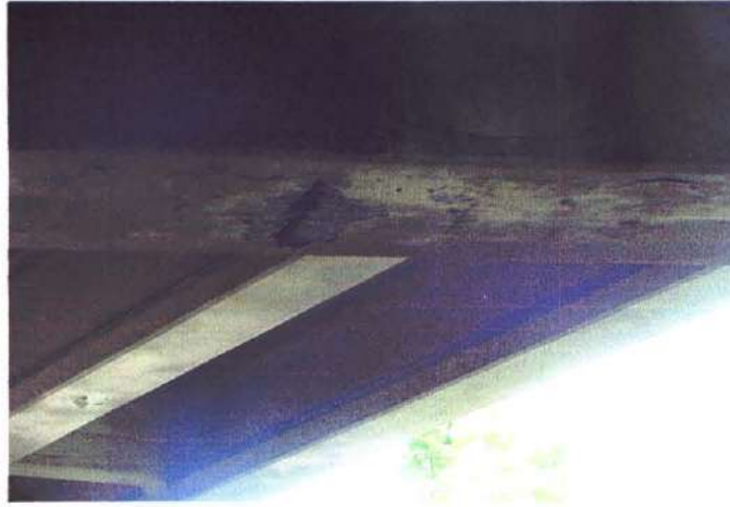
Spall & Rebar, Bottom of Bent Cap No. 1
