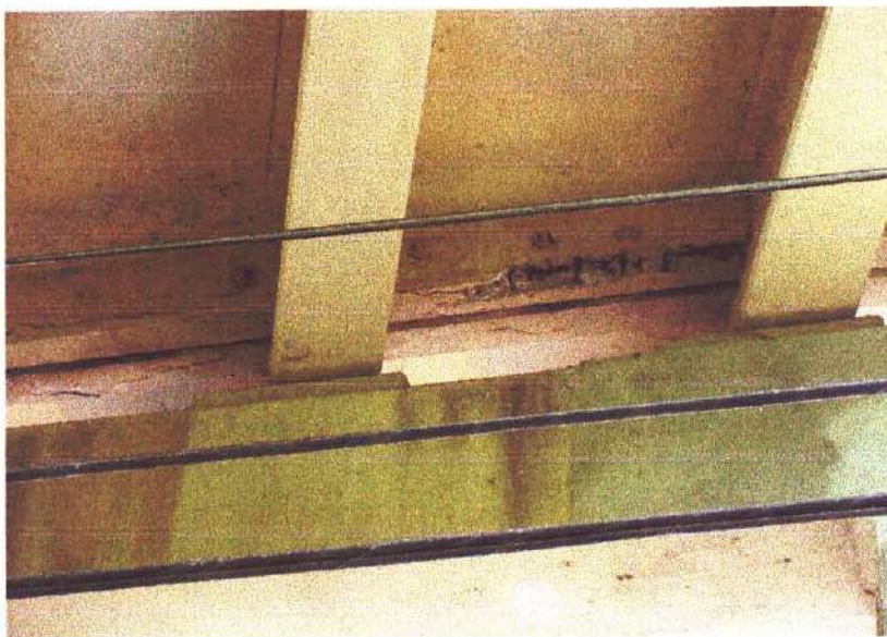
SPALL & REBAR IN DIAPHRAGM @ BENT NO. 2
