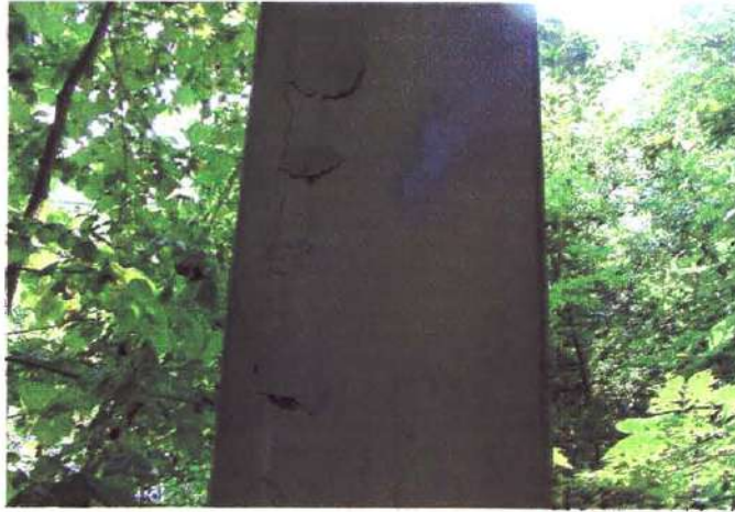
Cracks in Column "C" Bent No. 1
