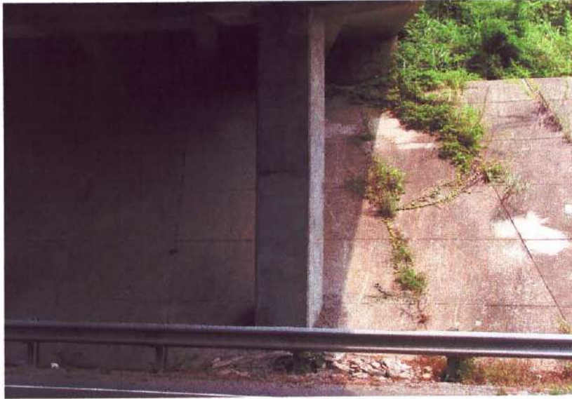
CRACKS, SPALL, & REBAR IN COLUMN "C", BENT NO. 3-REPAIRED
