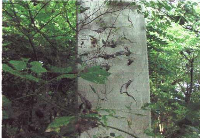
Cracks in Column "B" Bent No. 1
