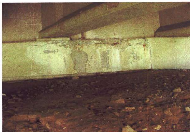
SPALL @ LT. SIDE OF ABUTMENT NO. 1
