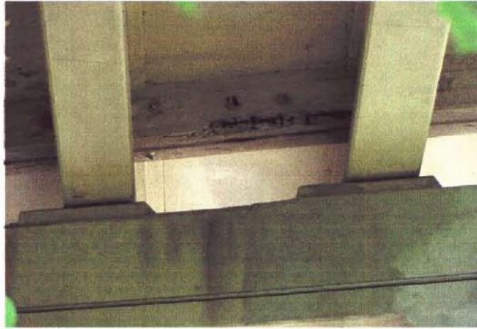
Spall & Rebar in Diaphragm @ Bent No.2
