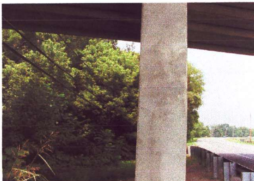
CRACKS, SPALL, & REBAR IN COLUMN "C", BENT NO. 2-REPAIRED
