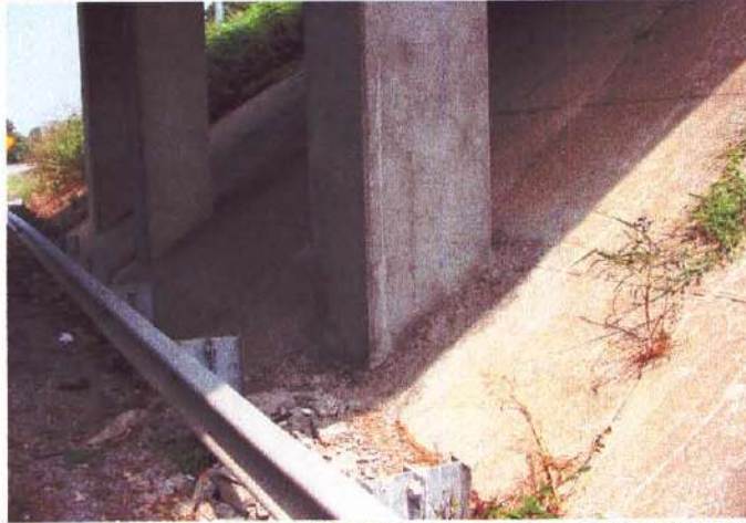
CRACKS & SPALL ON COLUMN "C", BENT NO. 3 @ BOTTOM (REPAIRED)
