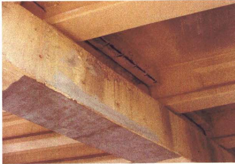
SPALL & REBAR IN DIAPHRAGM, BACK OF BENT NO. 3
